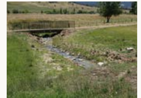
Poor drainage has impacted accessibility.
