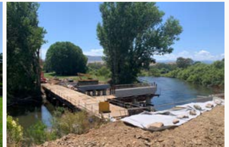
Proximity and access to the Murray River: the new Towong Bridge provides improved vehicular and pedestrian access.
