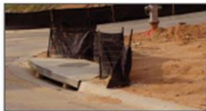
Figure 7. This silt fence doesn't work
