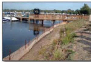
Figure 21. Silt fence protecting a lake shore
