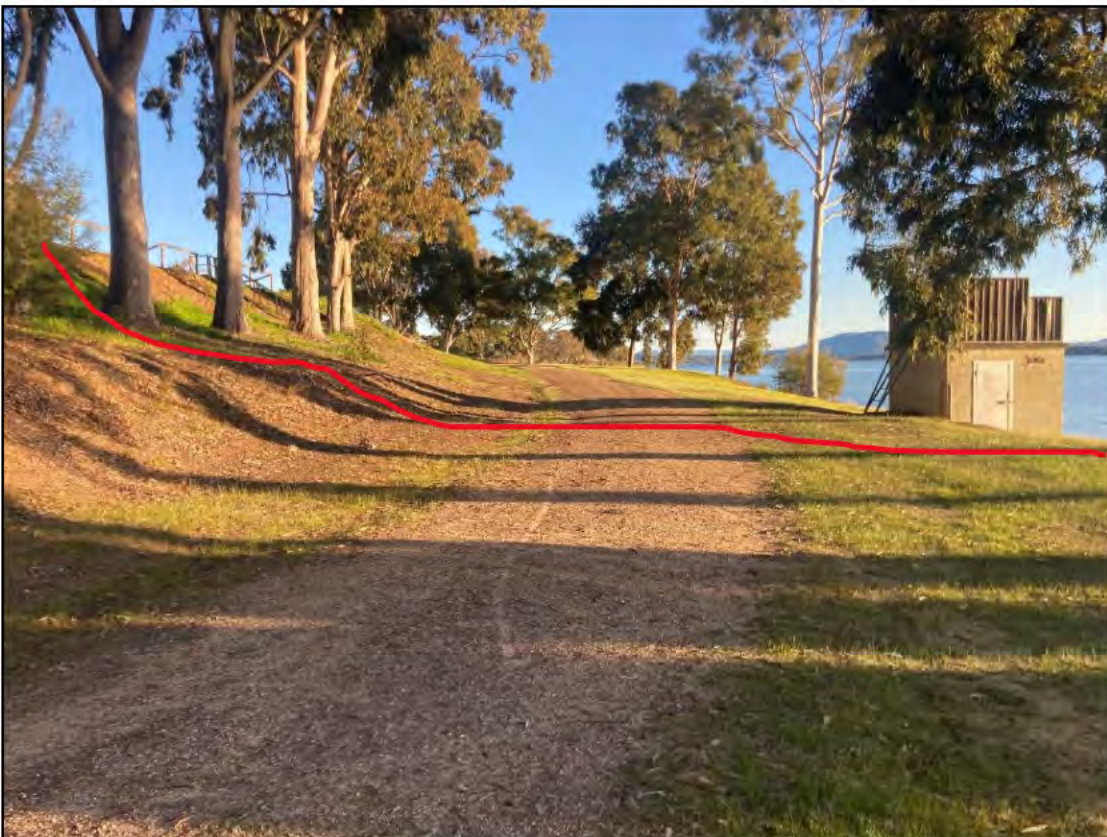
Photo 9: Imported gravel pathway, cut and fill. Very good to poor GSV. South orientation. D. Wall. 2022.
