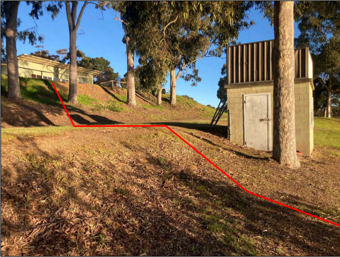
Photo 11: Existing utilities infrastructure, cut and fill. Poor to Good GSV. D. Wall. 2022.
