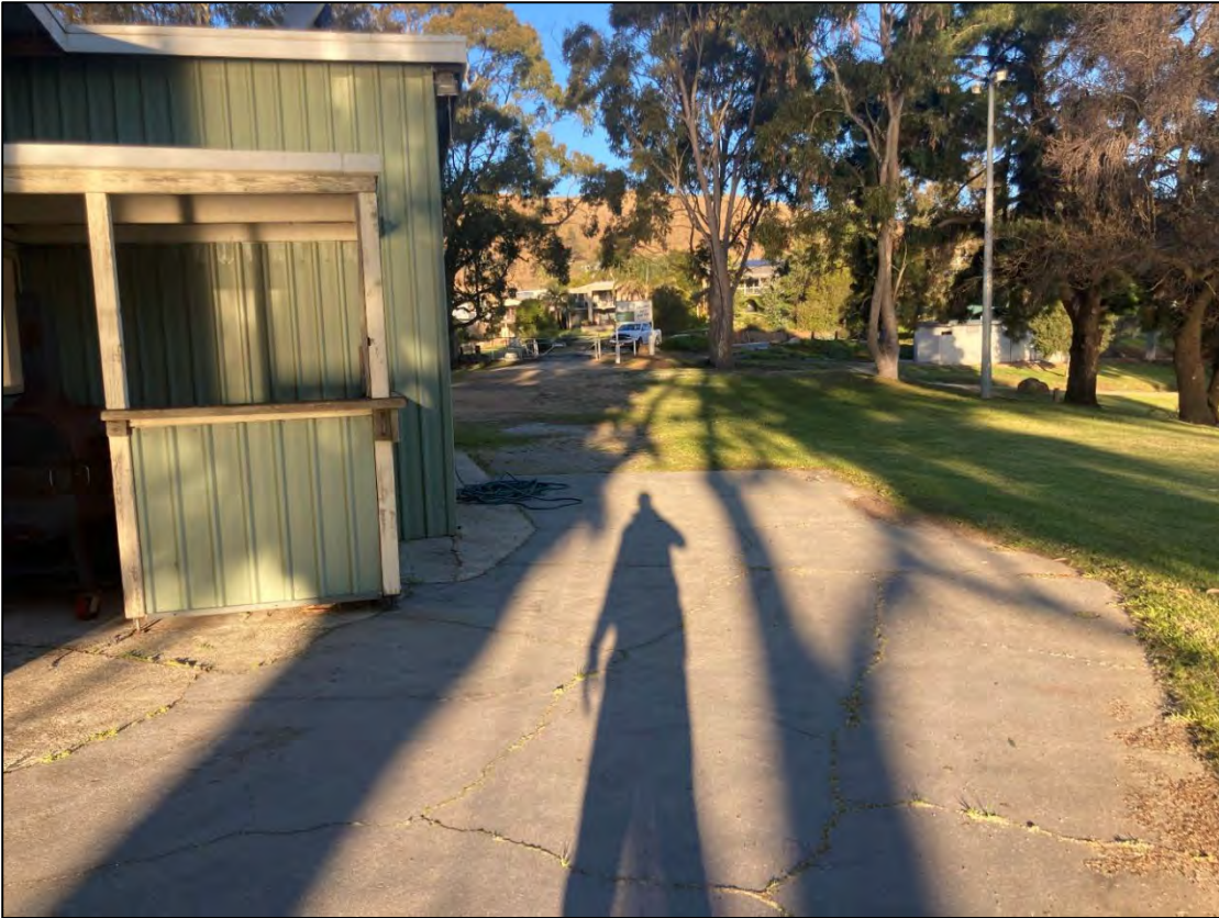
Photo 5: Concrete slab on the southern side of the Boat Club. Poor to no GSV. D. Wall. 2022.
