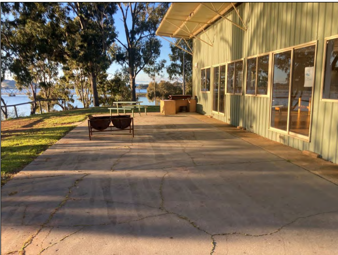
Photo 4: Concrete slab on the west side of the existing Lake Hume Boat Club. Poor to no GSV. North orientation. D. Wall. 2022.
