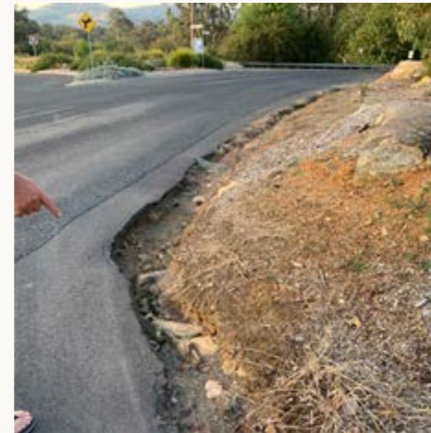
Damaged asphalt road surface on the south east approach to the bridge
