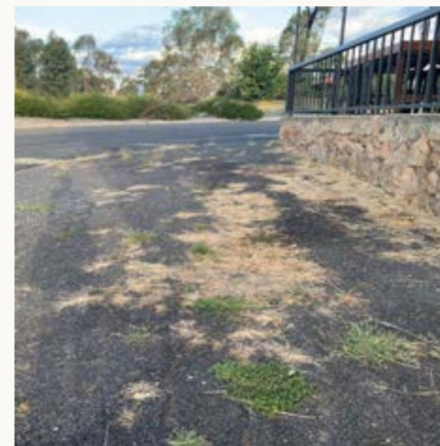
Condition of the footpath surrounding the Tintaldra Hotel
