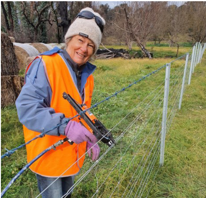
Picture: Blazeaid volunteers continue their work in the Towong Shire helping to rebuild burnt fencing.
