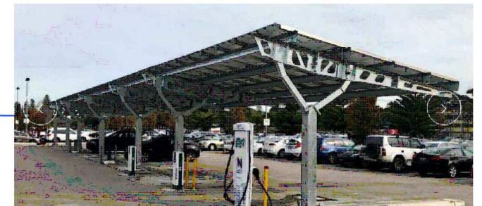
TYPICAL SOLAR SHADE STRUCTURE WITH EV CHARGER SUPPLY AND LAY UNDERGROUND ELECTRICAL CONDUIT TO HANSON STREET
